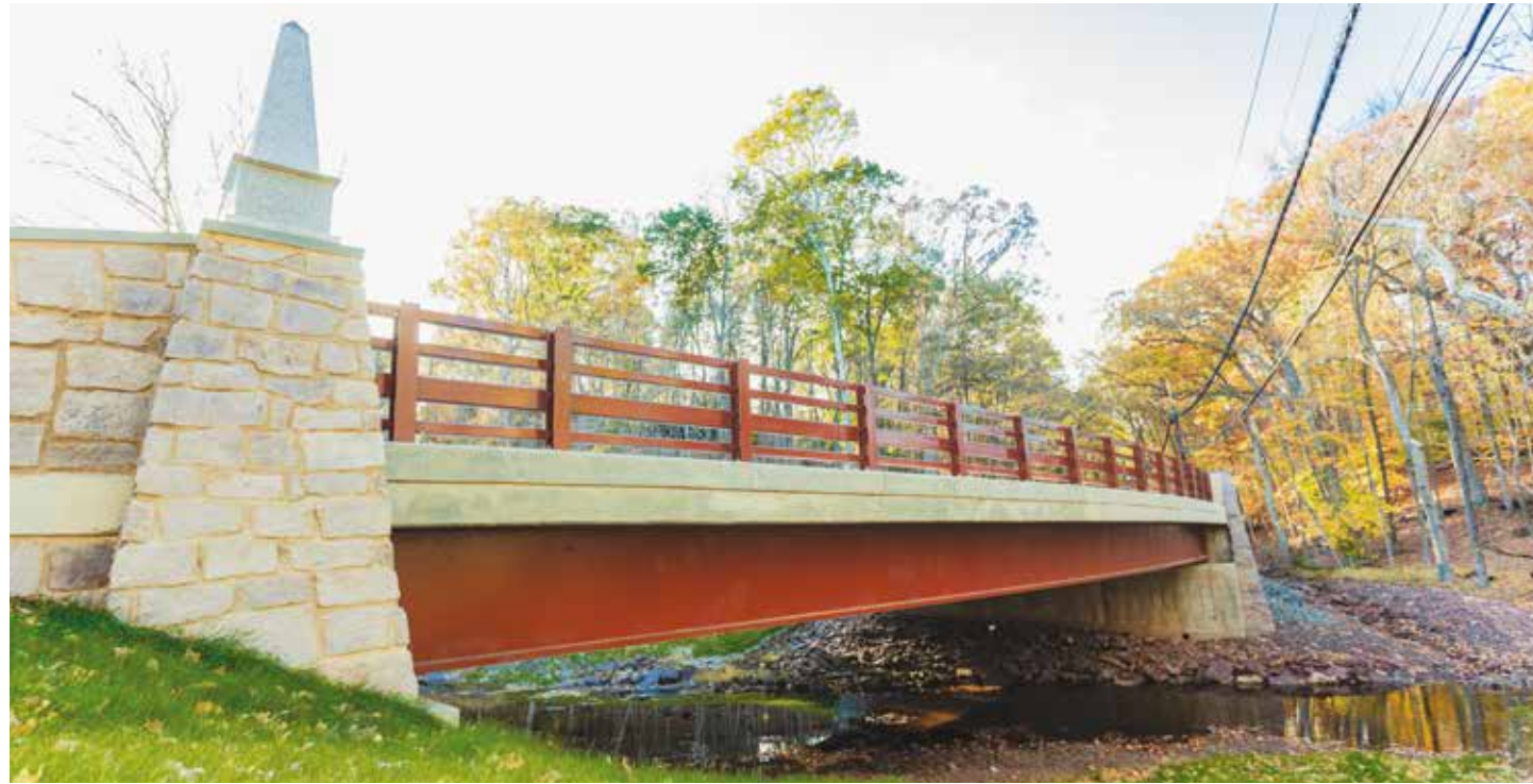
Bear Tavern Road and Jacobs Creek Road Bridges Mercer County, New Jersey Design
