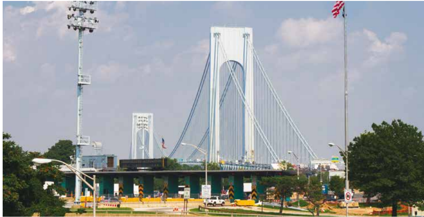
Verrazano-Narrows Bridge Brooklyn and Staten Island, New York Biennial and Special Inspections
