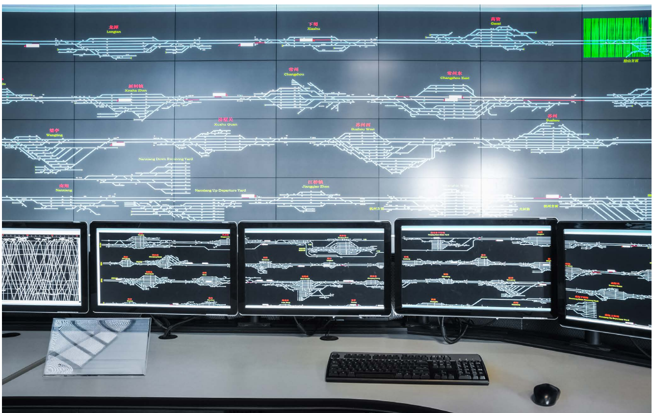
Figure 3: Control room digital network views (2D)
